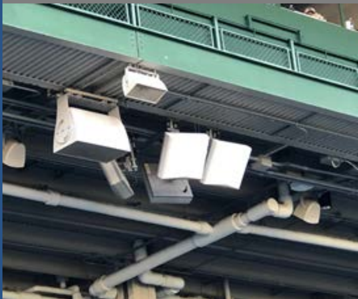
Extreme Networks Wi-Fi gear and JMA DAS antennas deployed by DAS Group Professionals cover the lower seating bowl from the upper-deck overhang.
